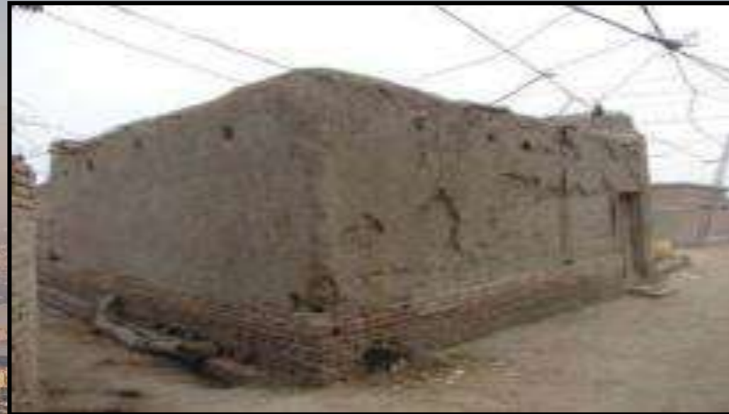
Poorly constructed Adobe Houses
