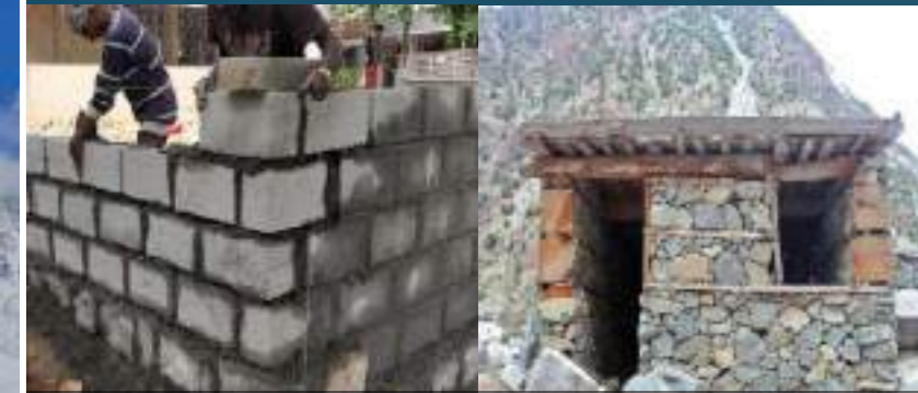
Poor Construction Practices
